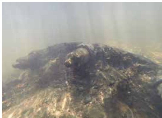
Exposed 24-inch CI flange under Raritan River
