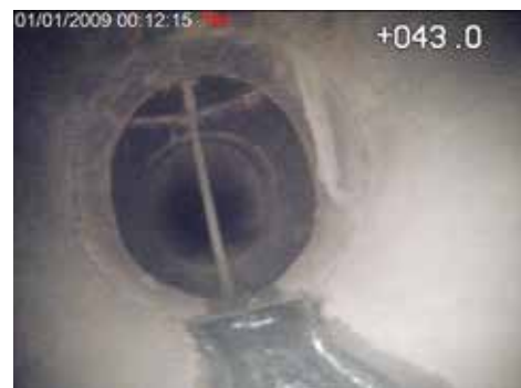
Unmapped drip pot identified by ULC crawler
