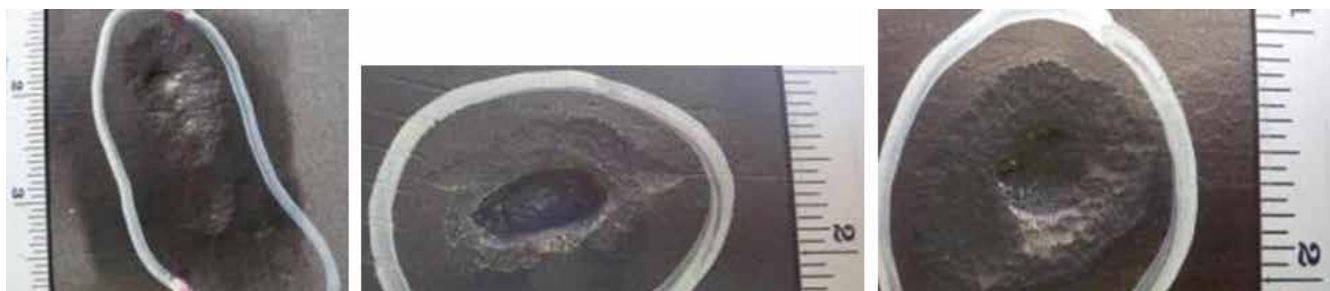
Figure 6. External metal loss anomalies
