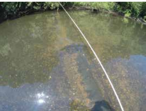
Exposed 24-inch CI main under Raritan River
