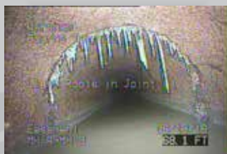
Roots at Joints
