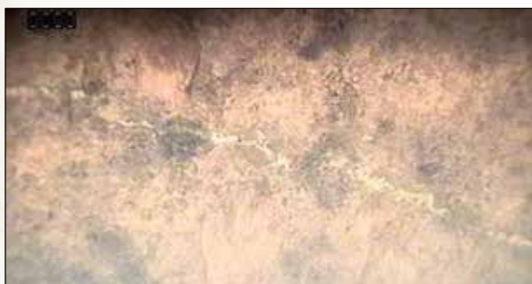
(a) Defect during 2011 ROV Inspection (SeaView, 2011).
