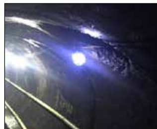
(b) Defect after dewatering.
