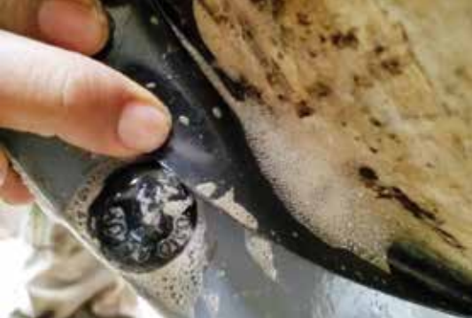
Leak at CI coupling
