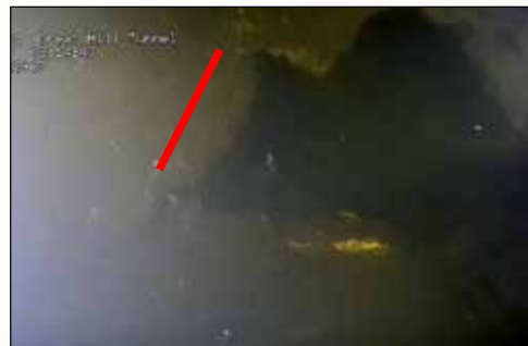
(b) Defect during 2017 Emergency ROV Inspection.
